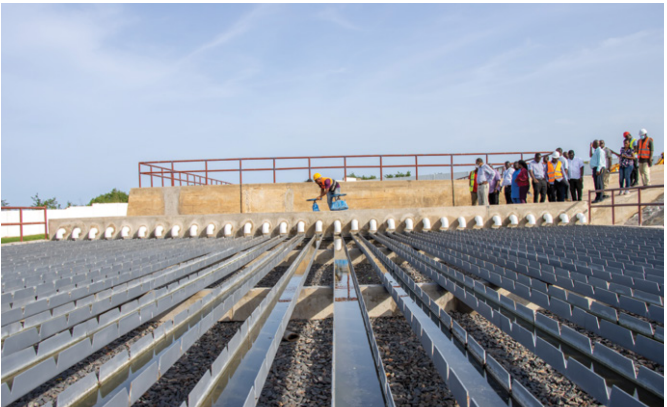
Trickling Filter at the Bankuman Facility
