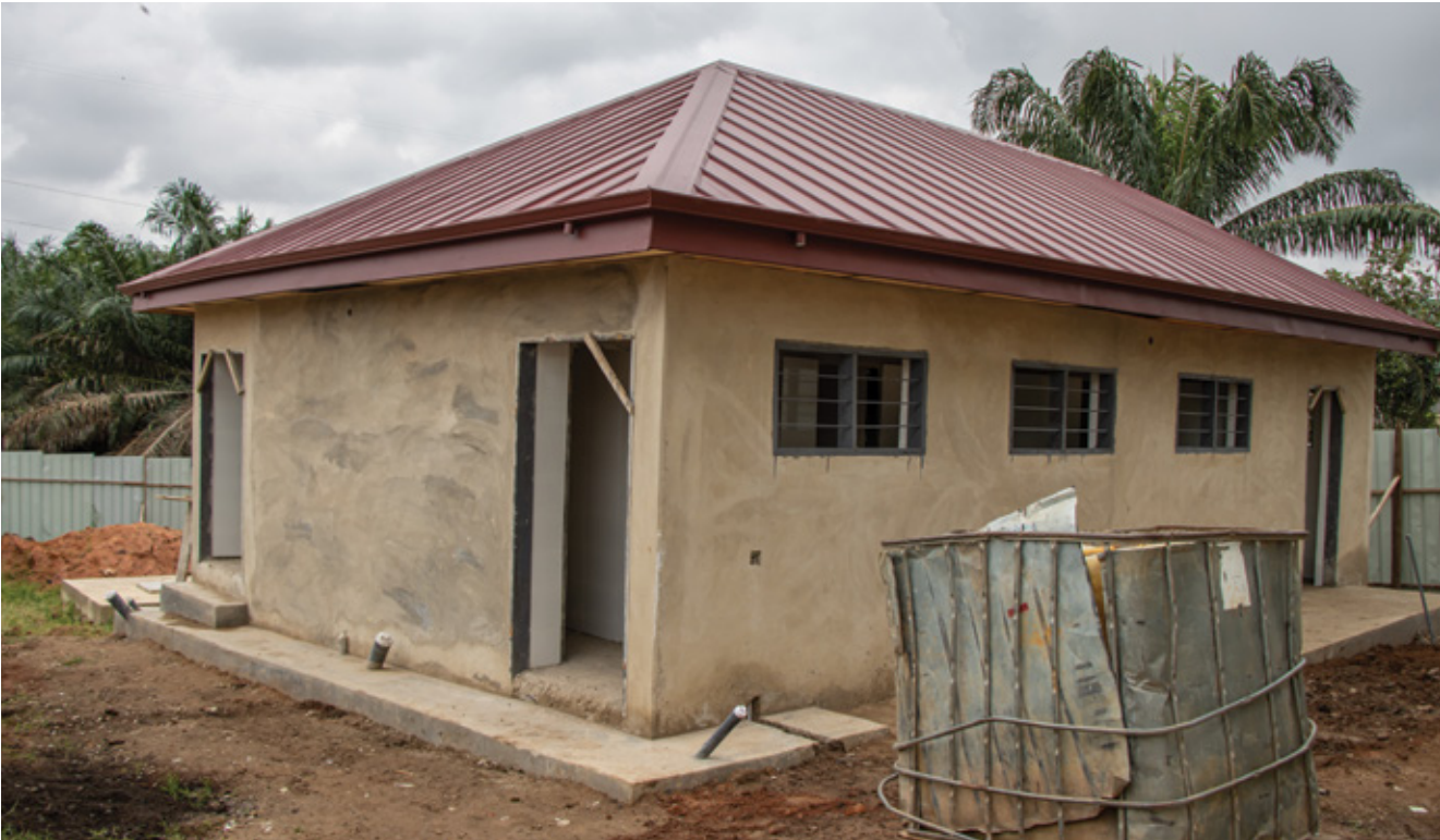
At school toilet almost completed at Kentinkrono in the Oforikrom Municipal Assembly
