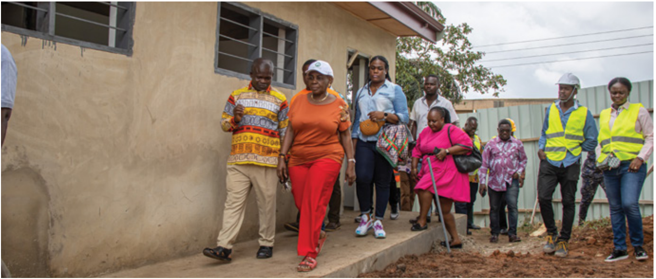
The Minister inspecting a school toilet under construction at Kentinkrono in the Oforikrom Municipal Assembly
