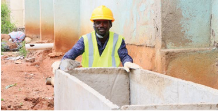
Figure 1 B: Photo of a biodigester installation.
