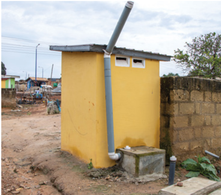
Figure 3: A stand-alone biodigester toilet
