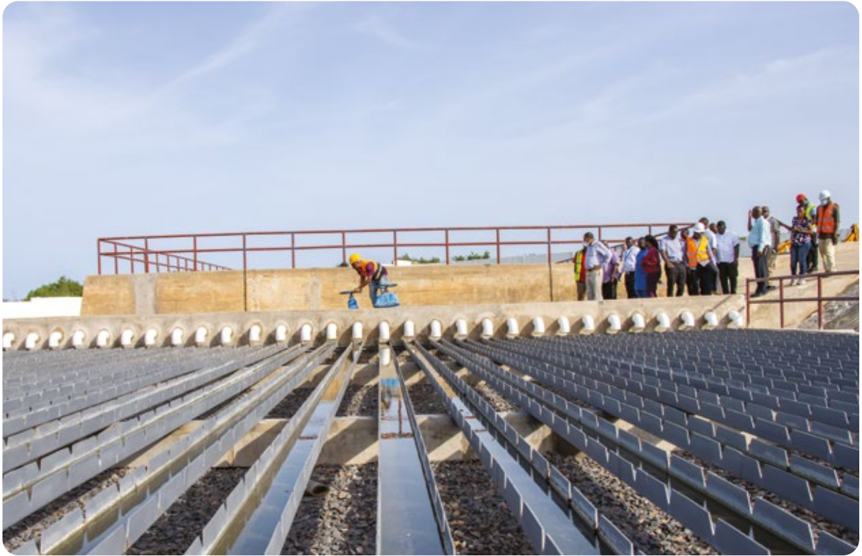
A World Bank monitoring visit to the Bankuman Sewerage Facility site during construction
